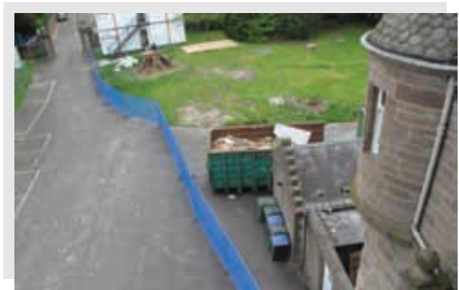
Demolition begins on the cottage to make way for the Castle Extension, 5 June 2012
