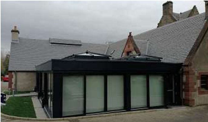
The new extension to the Cafe is nearing completion and will be opened on 26 April 2018.
